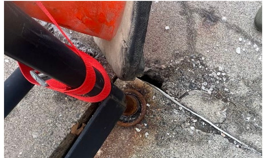
Hole in handicap ramp opened up on March 12 – through and through
